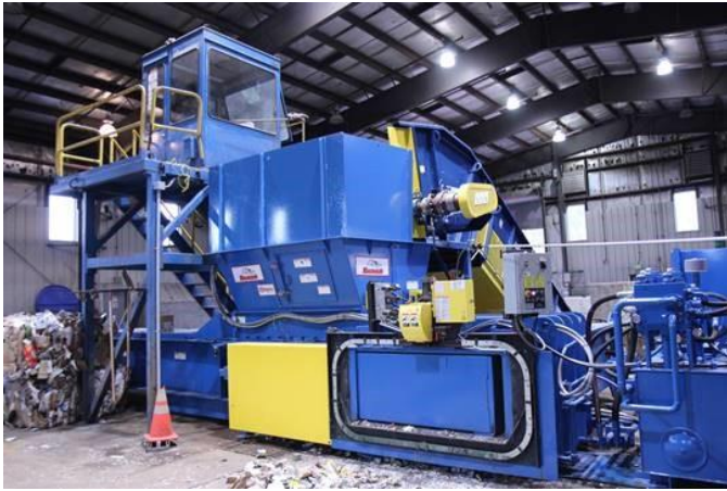
Figure 3: Baling machine located in Petersburg, AK.
