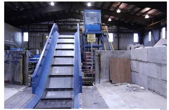
Figure 4: Conveyor belt attached to baling machine.
